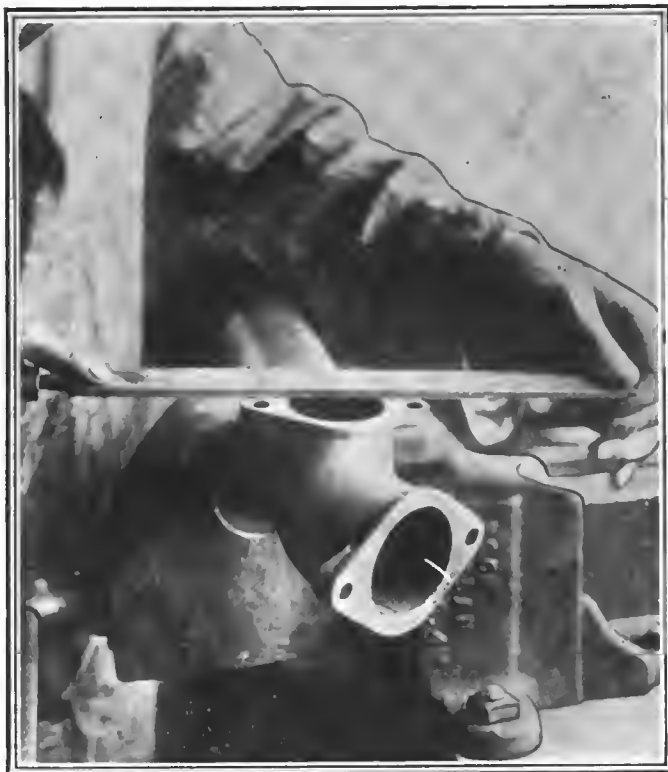
Fig. 1—Filing manifold flange to receive a new gasket properly, after the old one has been scraped off
